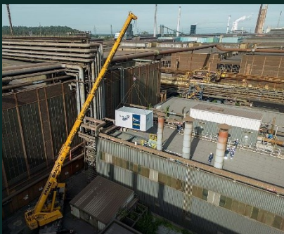
thyssenkrupp steel europe AG Power generation from waste heat
